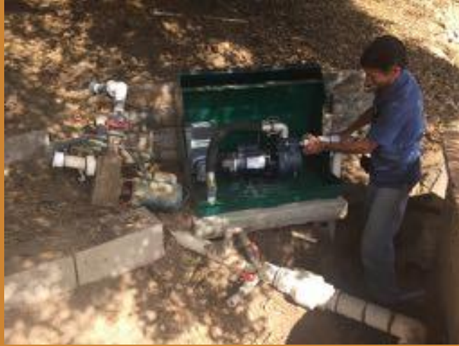
New and old booster pumps
